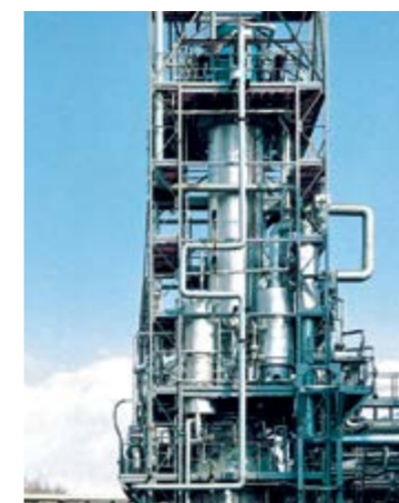
350 mtpd Methanol plant (grade AA) using innovative synthesis gas generation from waste products such as: clarifier sludge, used light and heavy oil, rubber waste, contaminated wood, and shredded material from recycling plants of motor vehicles. SVZ GmbH, Schwarze Pumpe, Germany
